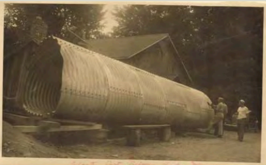
A view of the new culvert for the overflow from Damon's Pond on Damon Pond Rd. In Chesterfield, Mass.
